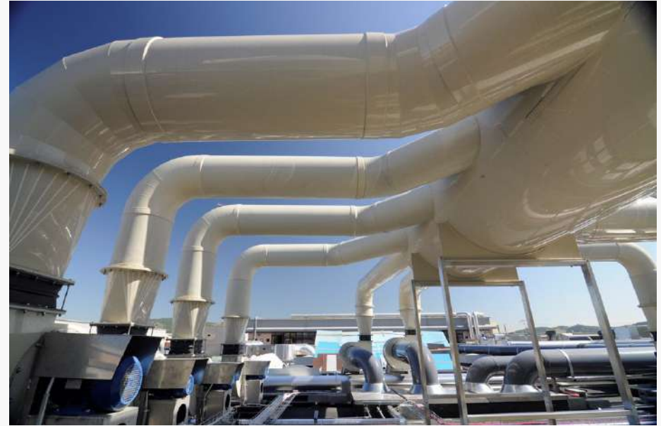
Sewage treatment plant - Pratella
